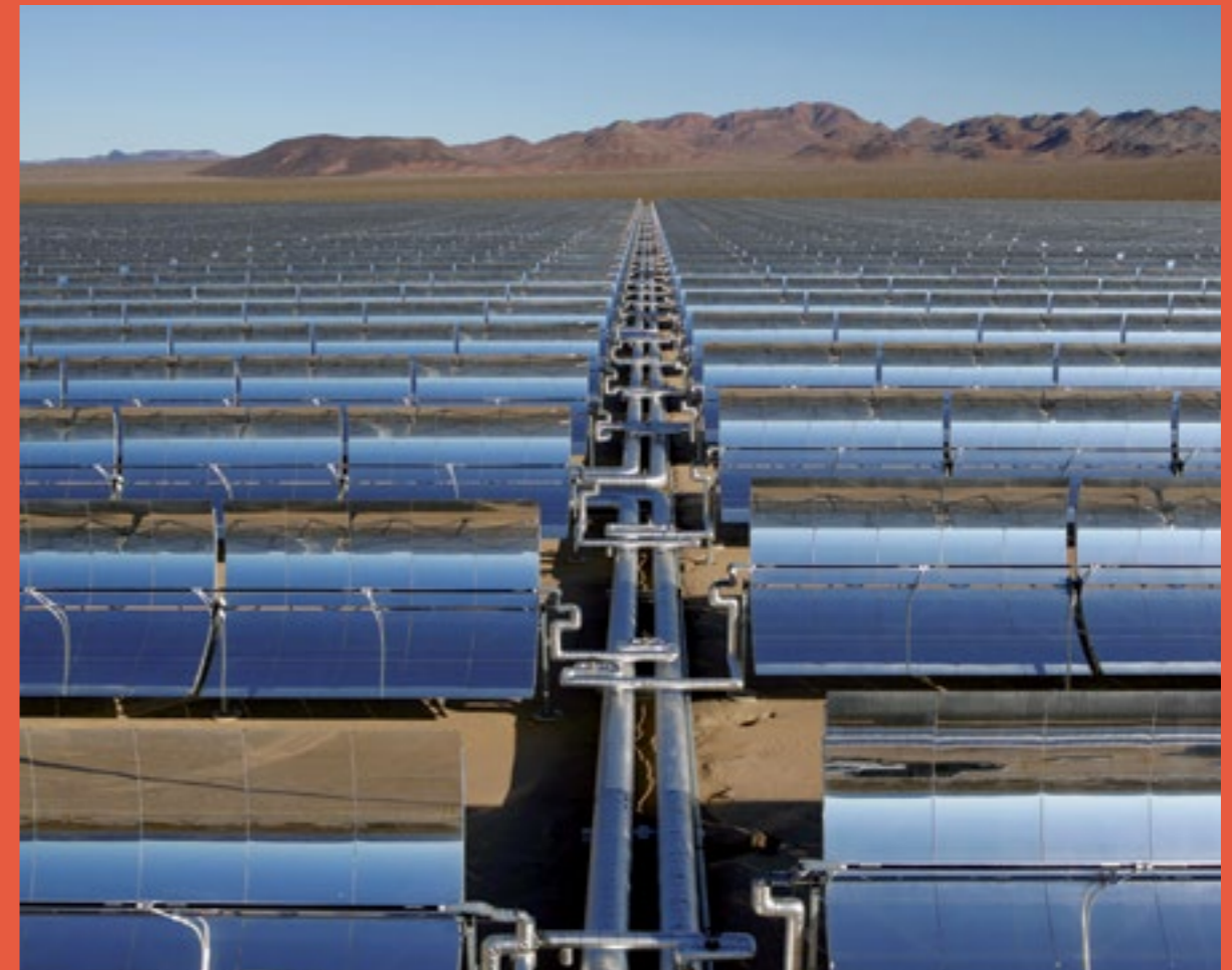
Solargenix Project 1, Nevada. Masdar Capital is invested in Solargenix
